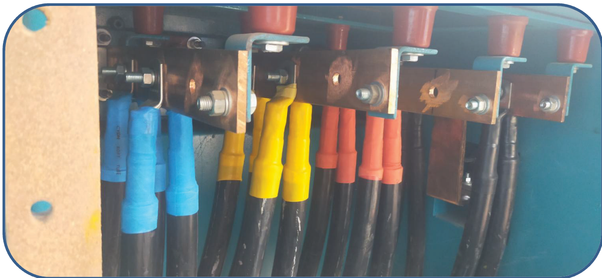
CABLE TERMINATION ON TRANSFORMER LV SIDE AT CCBU PREFORM & CLOSURE MANUFACTURE PROJECT 2022
