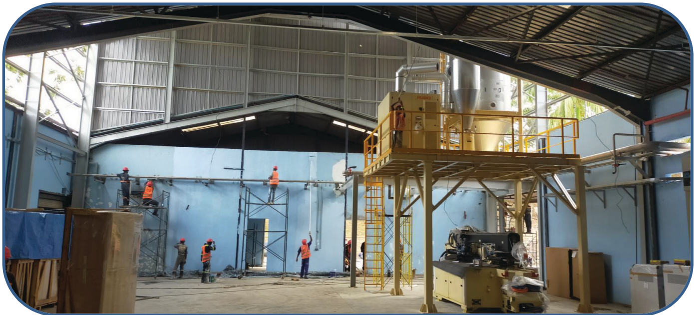
CCBU - RWENZORI - PREFORM & CLOSURE MANUFACTURE PROJECT IN 2022. WHERE EMFLO WAS AWARDED BOTH THE CIVIL & ELCTRICAL CONTRACTS WHICH WERE COMPLETED WELL AND IN TIME
