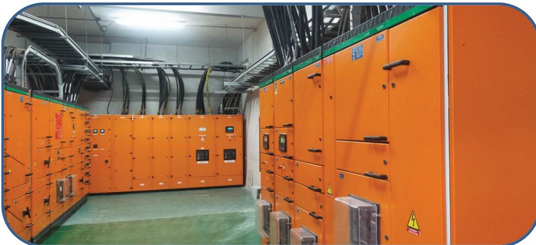
ELECTRICAL PANEL ROOM AT CCBU NEW PETLINE
