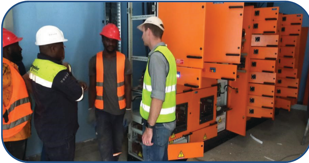
ELECTRICAL CONSULTANT ENG. NICO AND OTHERS DURING COMMISSIONING OF THE ELECTRICAL INSTALLATION FOR PREFORM & CLOSURE MANUFACTURING PROJECT
